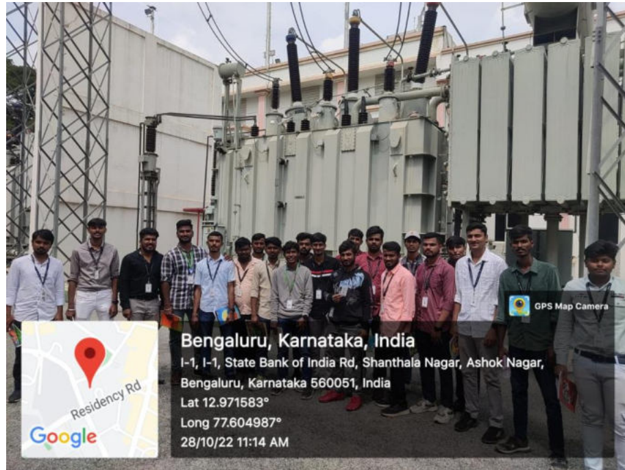
Fig. 1 5EEE students in front of 220kV/ 66 kV transformers at Sir. M.V East GIS, Bengaluru
