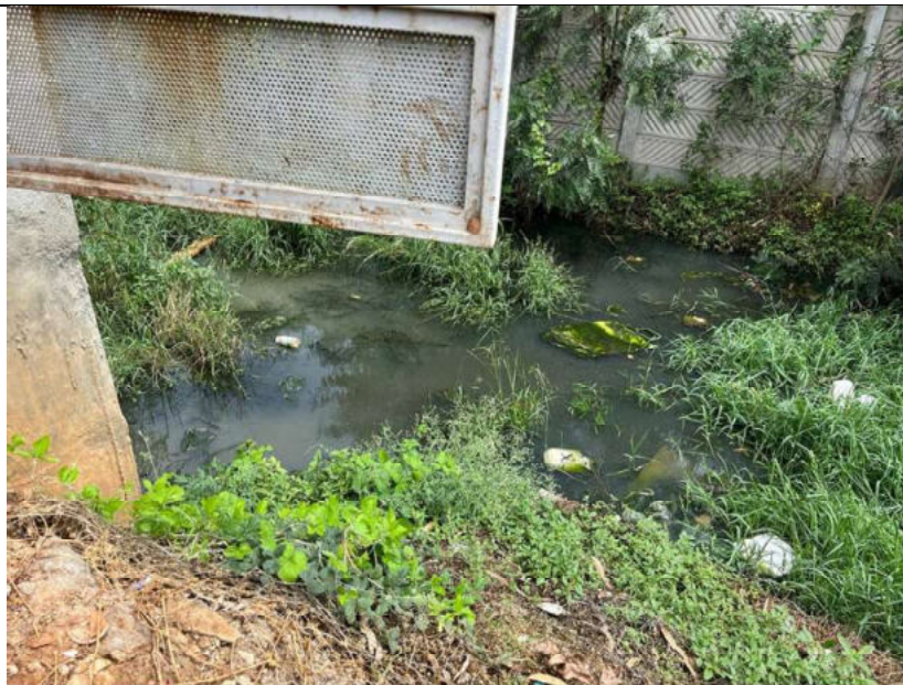
Sewage Treatment Plant out side (Presidency University, Bangalore, India)
