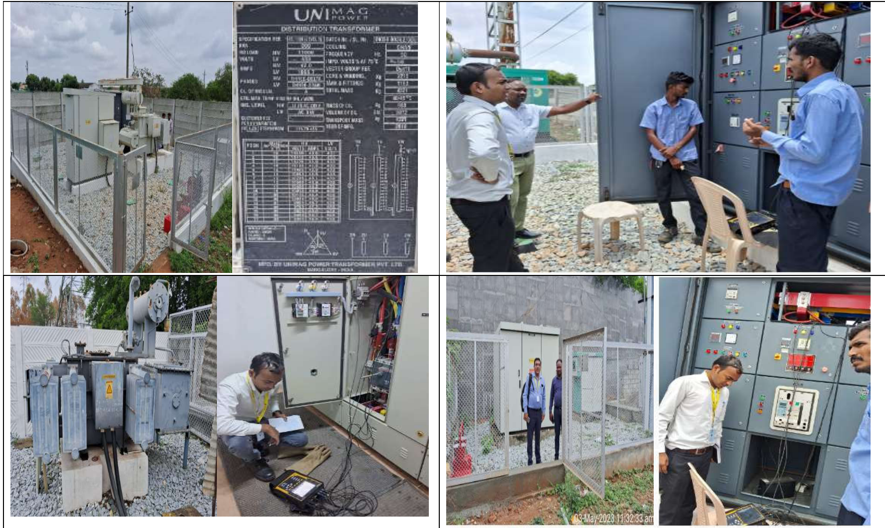
Figure 5: Site visit and measurement in transformer loading analysis
