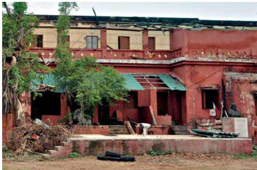
▲ FACELIFT AWAITED The dilapidated 'Pather Puri', once associated with Tagore
